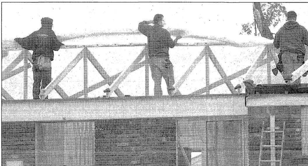
Monday morning at the Lake Pointe apartment complex, crews work to replace a roof blown away by Saturday's tornado.
