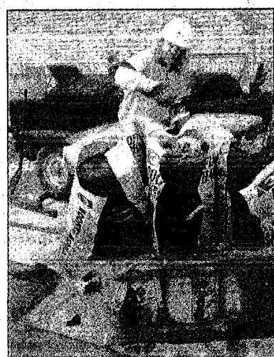
Dennis Baker of Fisher Roofing prepares materials for a new roof at the Plymouth Historical Museum.
