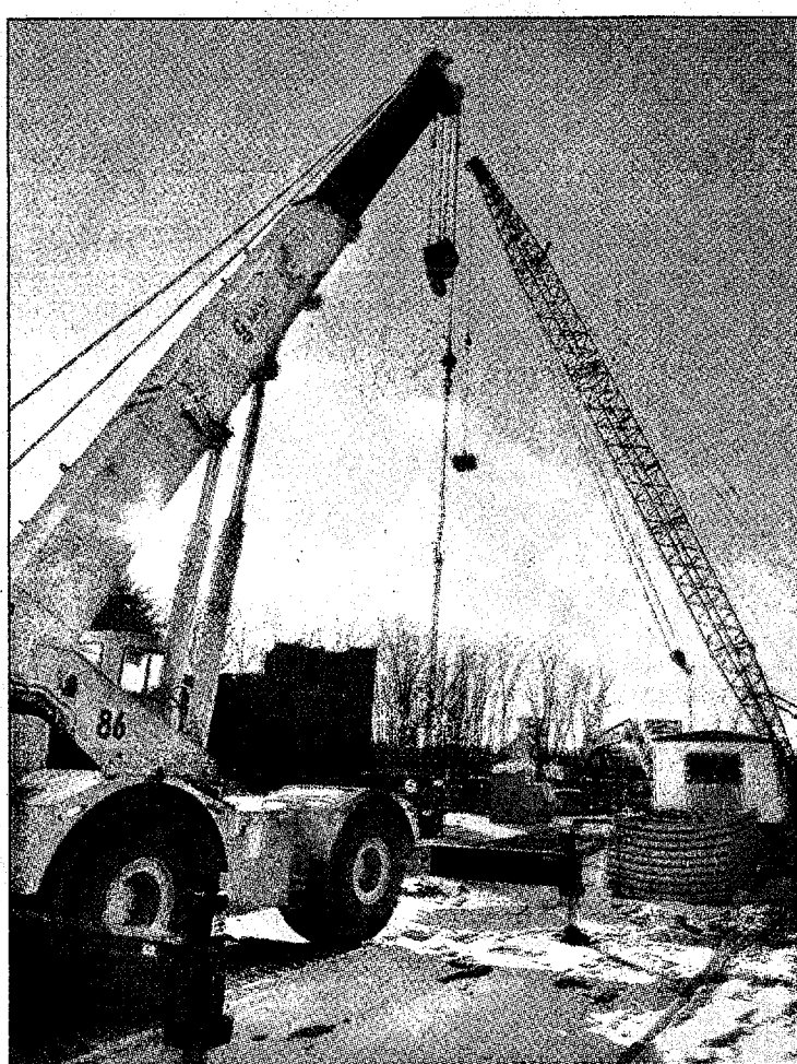
The end of a recent workday on the Sheldon underpass project, which is causing problems for businesses in the area.
