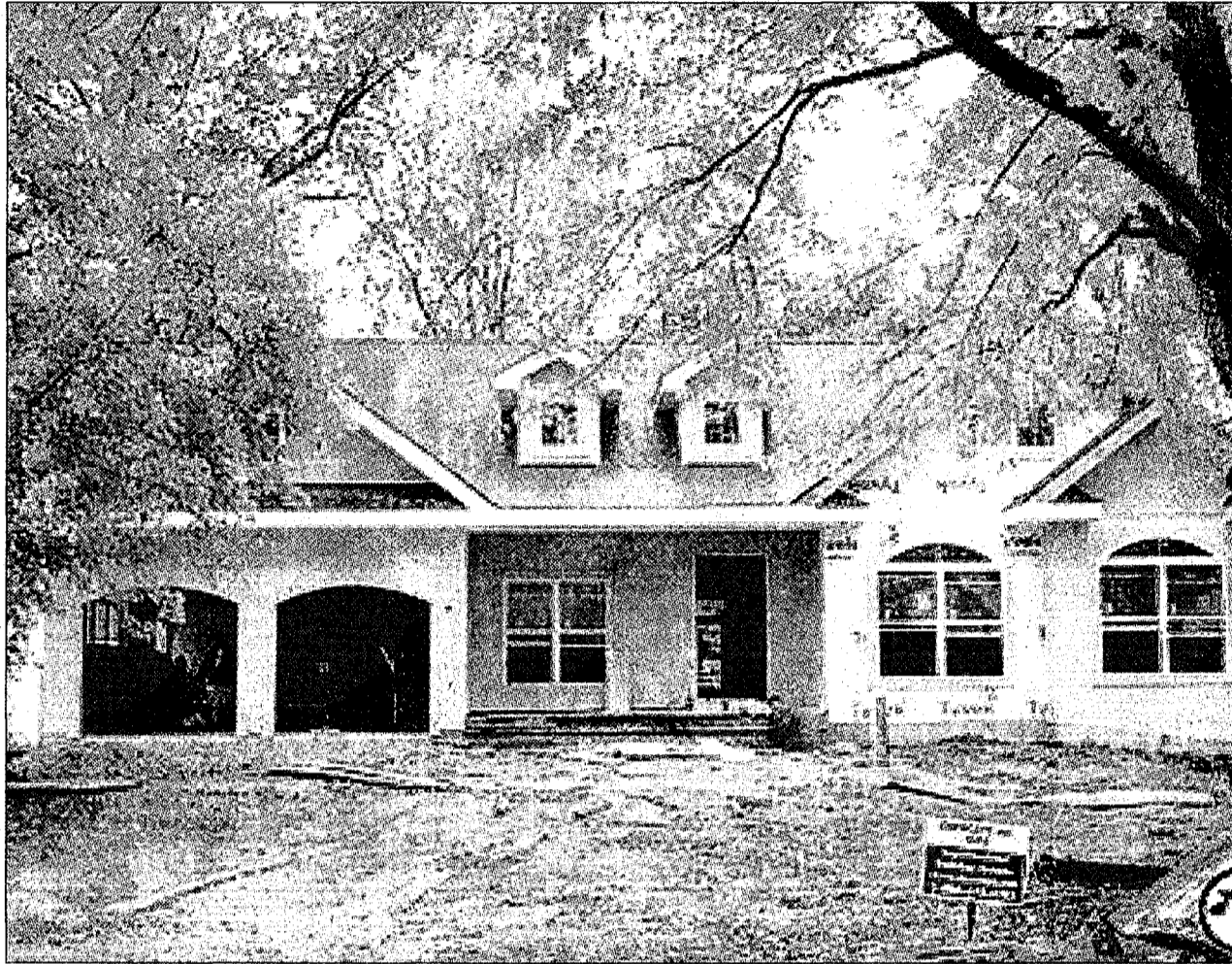
This green home is being constructed using energy-efficient and environmentally friendly building techniques.
