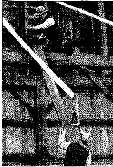
Amish workers are nearly done rebuilding the Cady Barn, which they disassembled and moved from its location on the Plymouth-Canton Educational Park.
