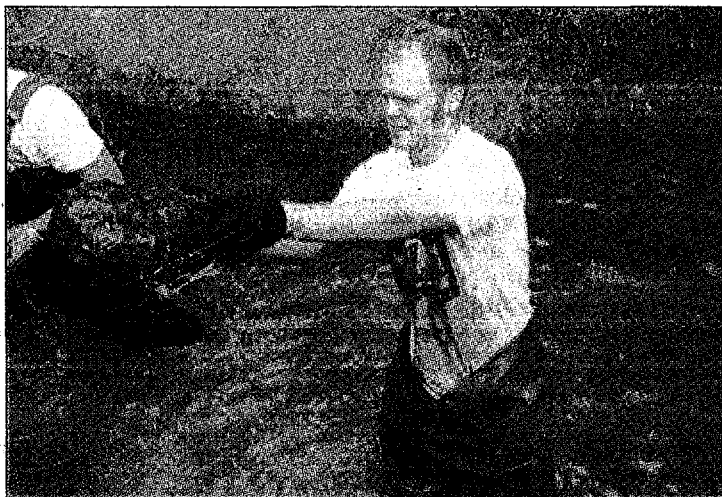
Schoolcraft Community College student Andy Brown helps remove rocks around the drain pipe at the Canton's Flodin Park.
