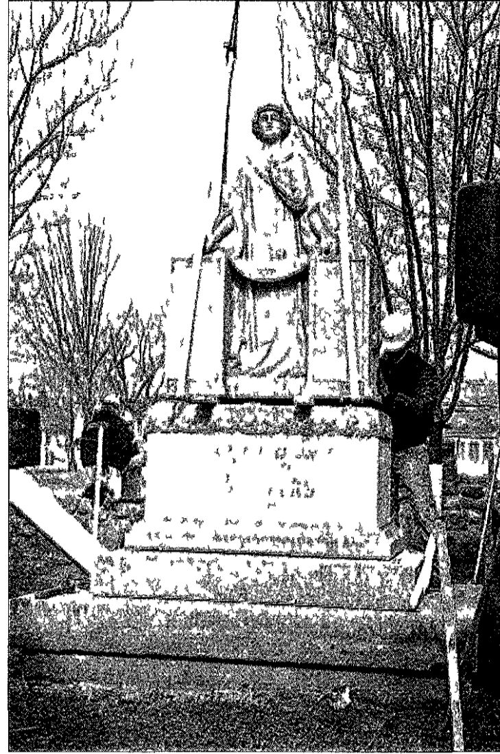
Workers place 'The Lady' on its base at the new Veterans Memorial Park being built in front of Central Middle School.
