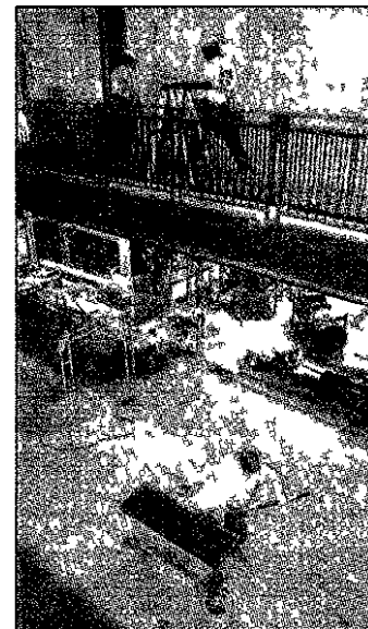
While the buildings at the new complex have been enclosed, work continues inside the new township offices.
