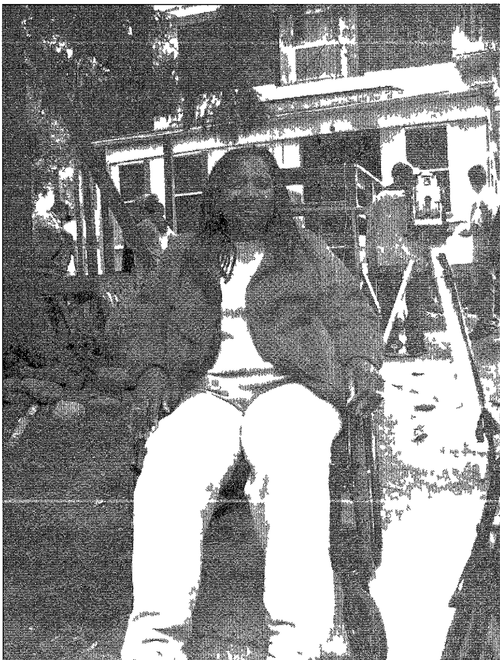
Sixteen employees from the Best Buy store in Westland work to complete a wheelchair ramp for Mary Donald of Inkster Donald became paralyzed from the chest down after undergoing spinal fusion surgery 3 years ago
