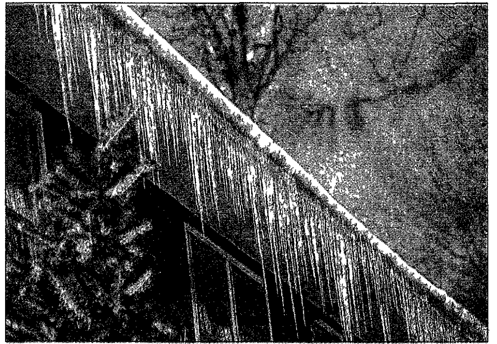
Don't let ice dams ruin your home. Prevent problems by taking action during the warmer months.
