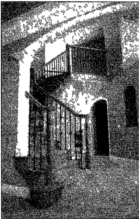
A stairway in a home under construction in Woodland Pond on North Territorial in Plymouth Township.
