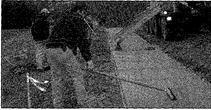
Crews put the finishing touches on sidewalks along Ann Arbor Trail near Plymouth Township Park as the 2003 sidewalk program comes to a close
