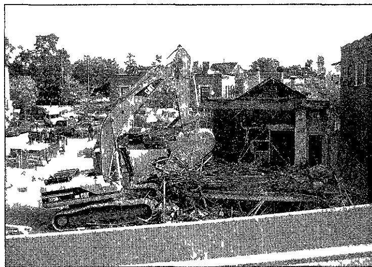
Bulldozers razed the Penniman Avenue building to make way for the long-awaited Tom's Oyster Bar.
