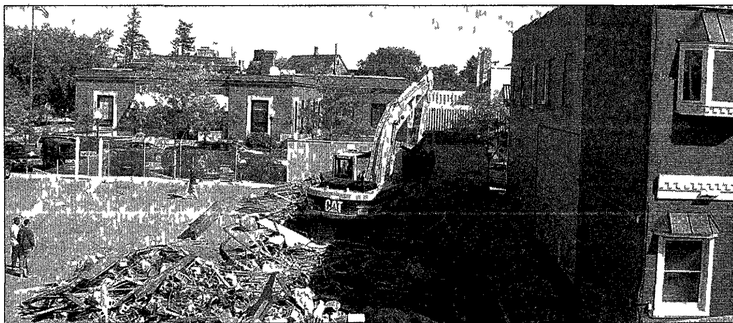
Is it possible we're actually going to see the Oyster Bar downtown, after years of anticipation? The old building is down now, with construction slated to start soon on the new one.
