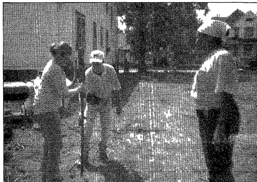
Chris Stenquist and Jerry Grodsky help a Habitat volunteer and home recipient install a fence.
