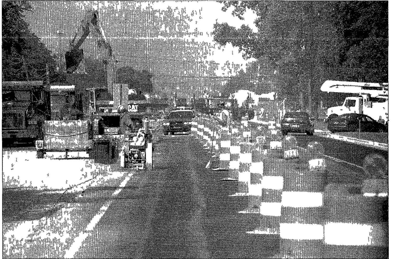
Orange barrels have been a familiar sight along Ann Arbor Road this summer. The eastbound lanes are coming along ahead of schedule though, according to a worker on site Friday. PAUL HURSCHMANN(OBSERVER)
