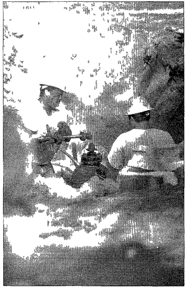
Construction workers install a water main along Penniman at Church. PAUL HURSCHMANN(OBSERVER)
