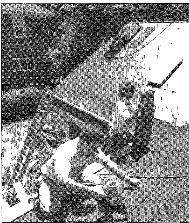
Roofers Chris Bates, Kenny Satterlee and Don Lee from Classic Builders Inc work on the Kiwanis project home
