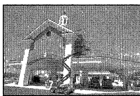
Facade finishing: Workers put the final touches to the front of one of the colonial-style buildings that make up the Plymouth Super Center
