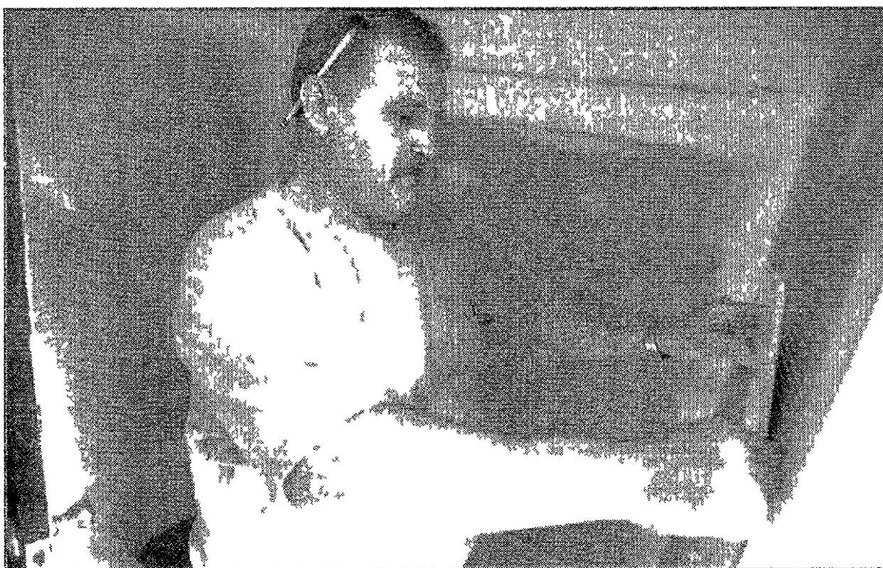
Fix it up: Richard "Lefty" Frizzell first drywalled, then installed new tile.
