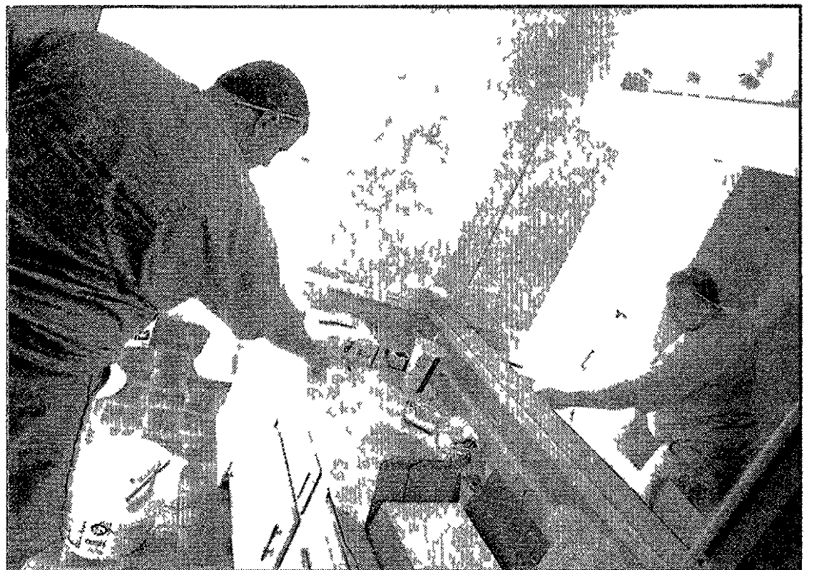
From bad to good: Frizzell also installed a new sink and countertop as part of the remodeling project.
