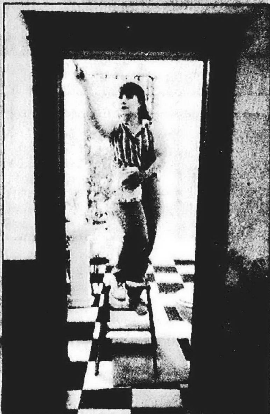
Restoring: Valerie Skowronek paints the trim around the doorway of a bathroom just outside the kitchen. In the foreground you can see the detailed wood trim and original wainscoting.
