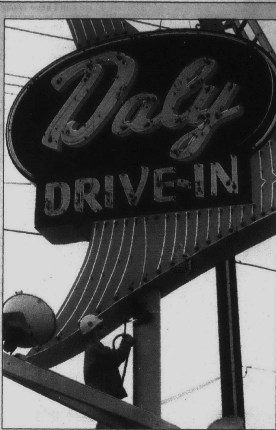
Goodbye Daly's: Matt Wilson uses an acetylene torch to cut through the double steel post holding up the Daly's sign on the northwest corner of Main and Ann Arbor Road Friday. Patrick Gallagher of Furniture Restoration Station in Plymouth purchased the sign at auction. He'll keep half of it and plans to donate the other to the museum.
