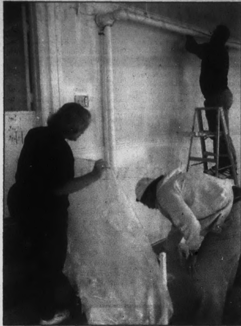
Careful aim: Marie Lamberg holds a plastic sheet as a shield while her husband, Cliff, applies white spray paint on a railing to stairs leading into the dining room.
