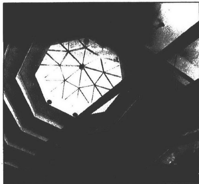
An octagon-shaped skylight over a glass escalator (shown in foreground under construction) highlights the new 150,000-square-foot Laurel Park store.
