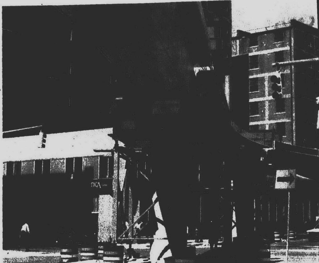
This is a section of the elevated rail people mover system in downtown Detroit. Plans called for all beams to be in place by winter with the system operating in 1986.
