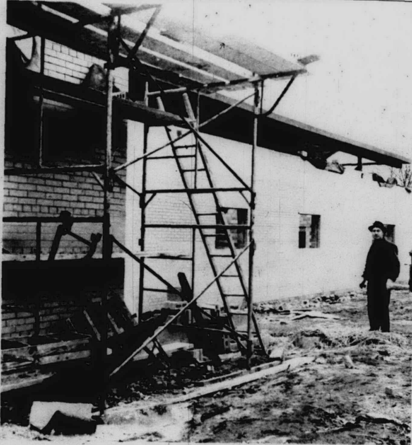
PROGRESS IN Bill and Dean Saxton's new Garden Center building was being noted this week as builders awaited steel stringers and rafters for the roof. Saxton's, located on Ann Arbor Trail near Kellogg Park, announced expansion plans last fall that called for a doubling of present floor space (up to 11,300 sq. ft.) and increased parking spaces. Saxton, here in front, said last week he hopes to have the building done by March.
