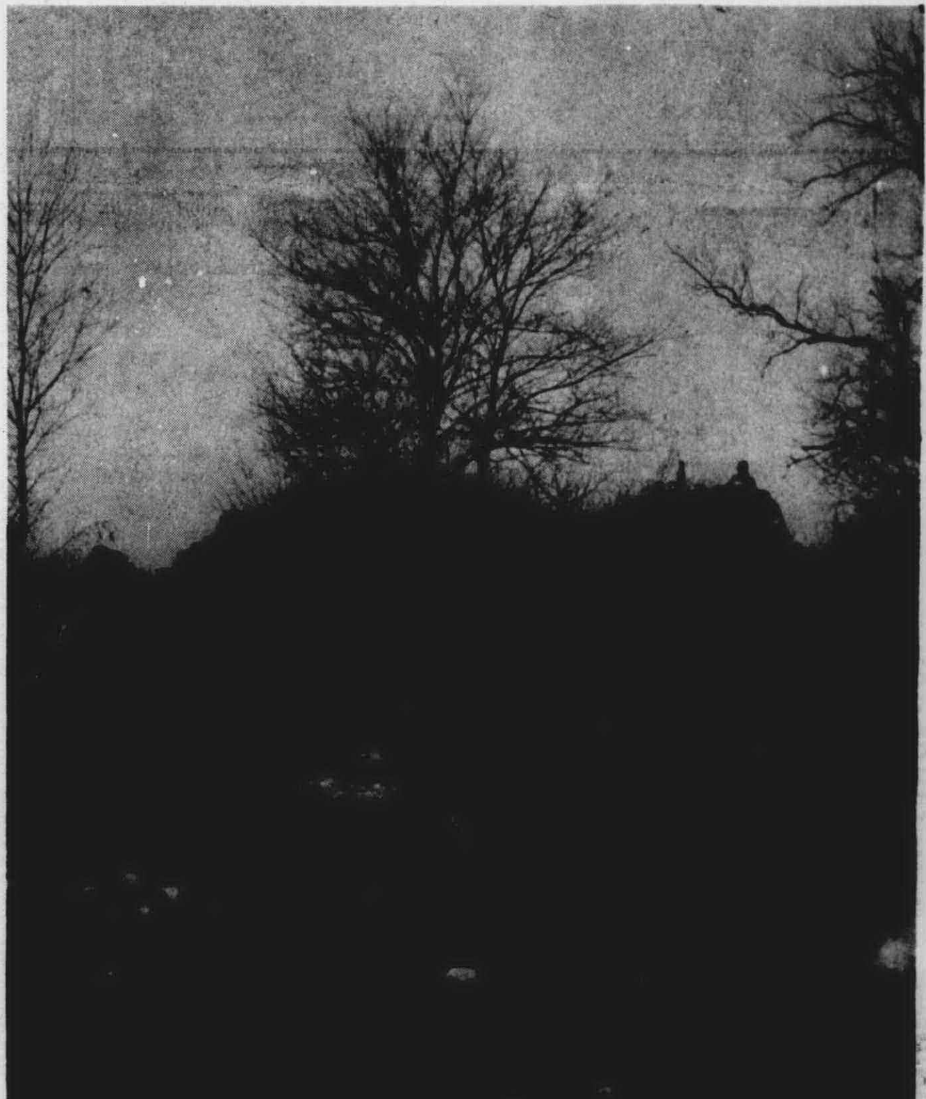
A GAPING HOLE in the earth-work of the dam shows where the artificial lake poured through last Sunday. A tractor atop the dam was busy at work Monday morning fixing the damage. The lake was on the other side of the dam shown here.
