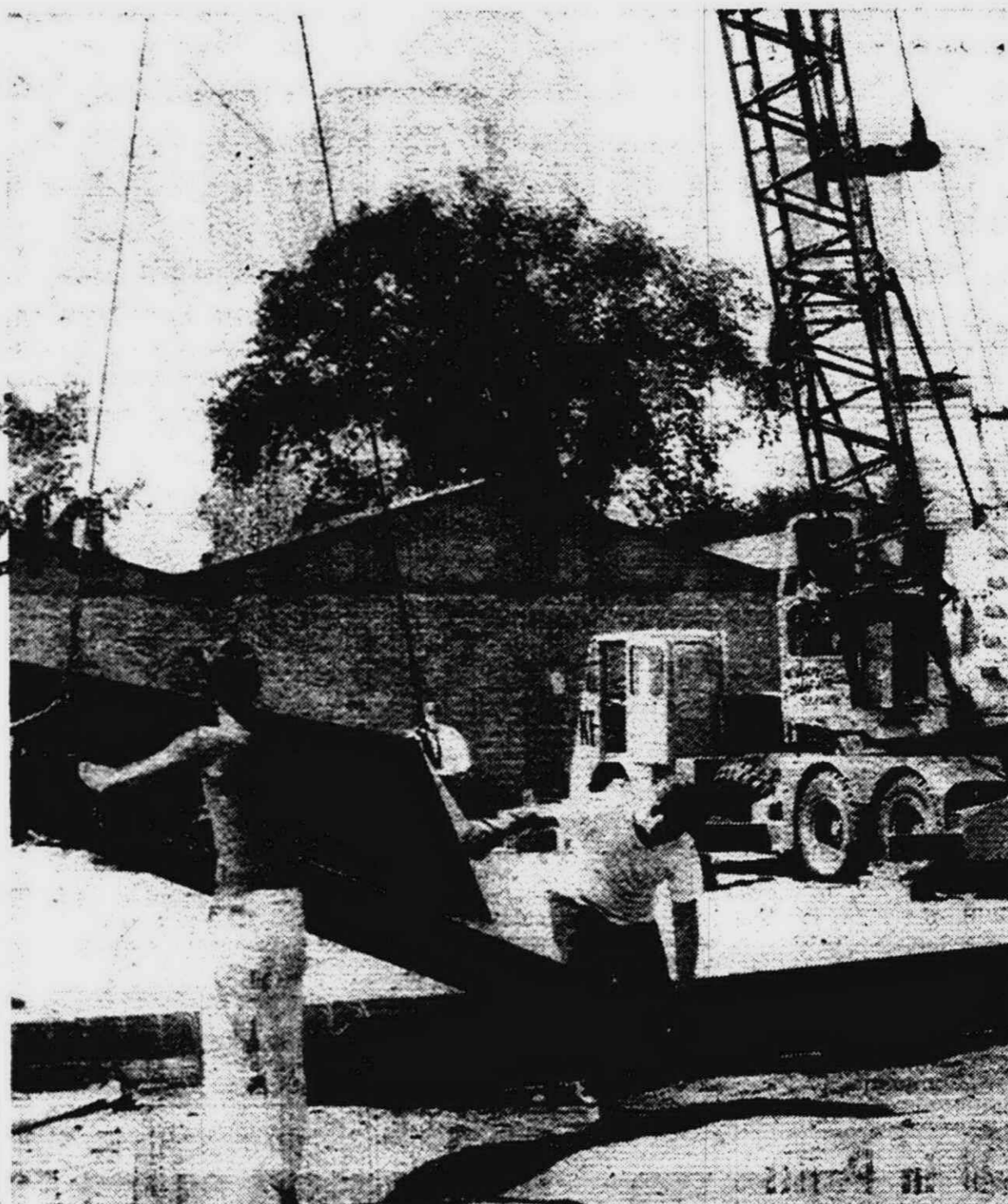
WORKMEN BEGAN unloading steel Monday morning at the site of the new addition to D.S.I. Corporation's plant in Plymouth. Structural steel on the project is expected to be erected by the end of this week, according to W. C. Scott, president. Plymouth's Industrial Development Corporation will launch a drive soon to raise more than $34,000 in funds to help finance the project.
