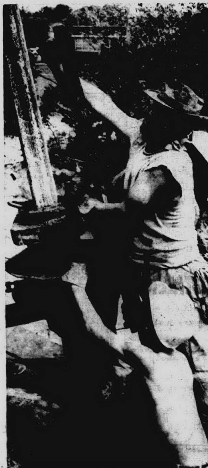
WORKERS AT new drilling site get set to sink well some 4,600 feet into the ground.
