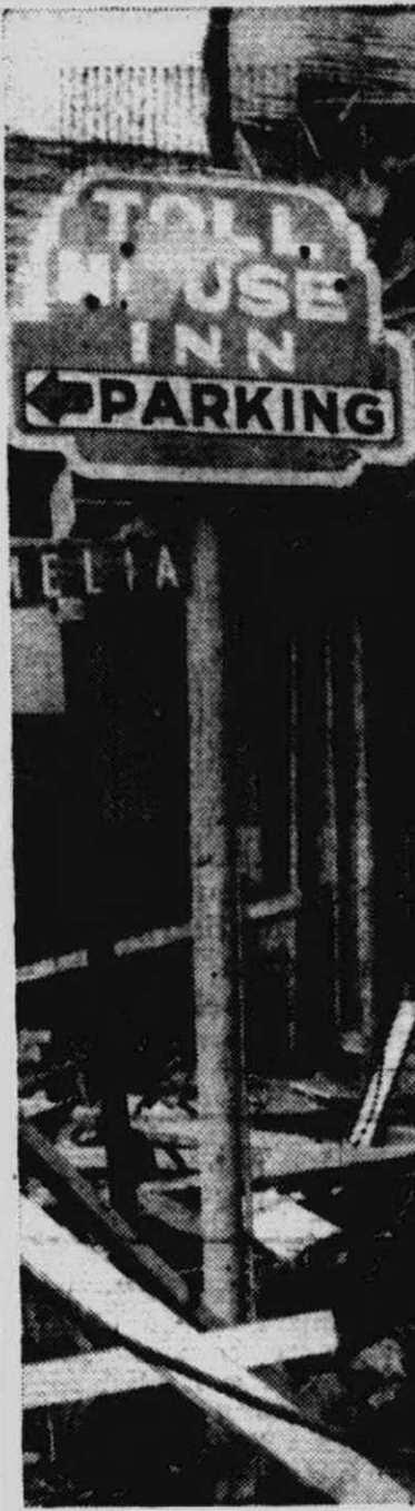
TOLL HOUSE Inn, a favorite dining spot for many Plymouthites over the years, is being torn down this month to make way for a parking lot for Allison Chevrolet dealership.
