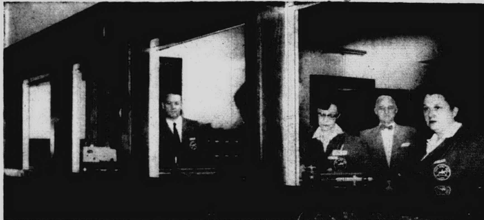
THE LOBBY in Plymouth's post office is sporting a new look these days. Work recently was completed on the installation of new aluminum shuttered windows, new counter tops and lock boxes. Shown behind the remodeled teller windows are postal employees Fred Carter, Mar-
