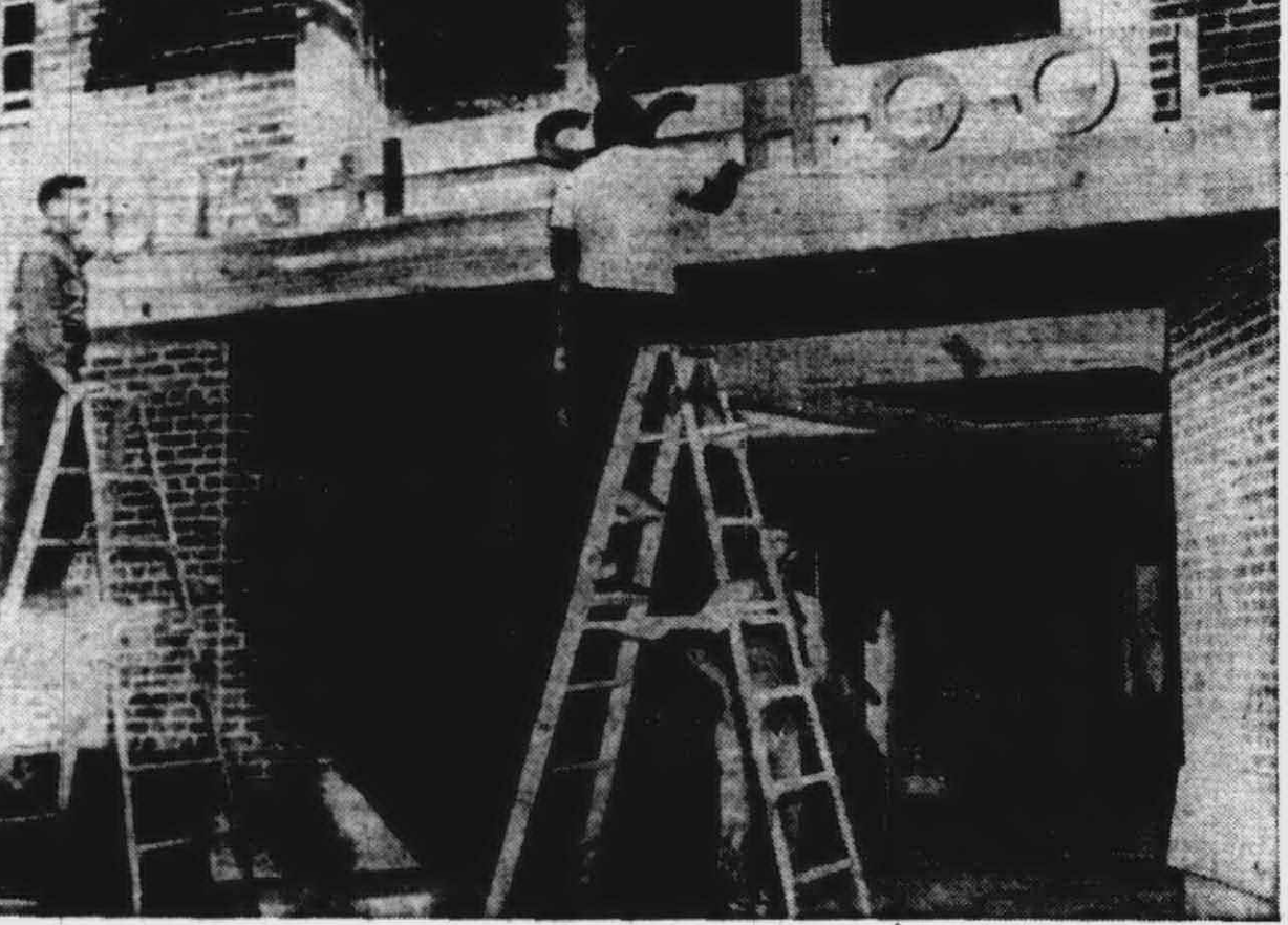
THE WORDS "High School" were erected Tuesday noon on the new Senior High entrance as workmen rushed to complete over a quarter million dollars worth of construction in the building. A new stair tower has been erected on the building's front, one of several projects demanded by the State Fire Marshal's office.
