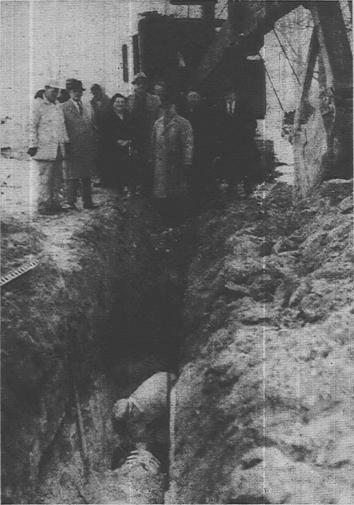
THE FIRST SECTION of water main for Plymouth Township's $1,100,000 water expansion program was laid Monday morning and on hand to take part in the occasion were Township officials. The first water main was laid on Schoolcraft Rd. near Fire Station No. 2. It will hook into the Detroit water main at Eckles Rd. and then into the present Township system in Lake Pointe Village. By
