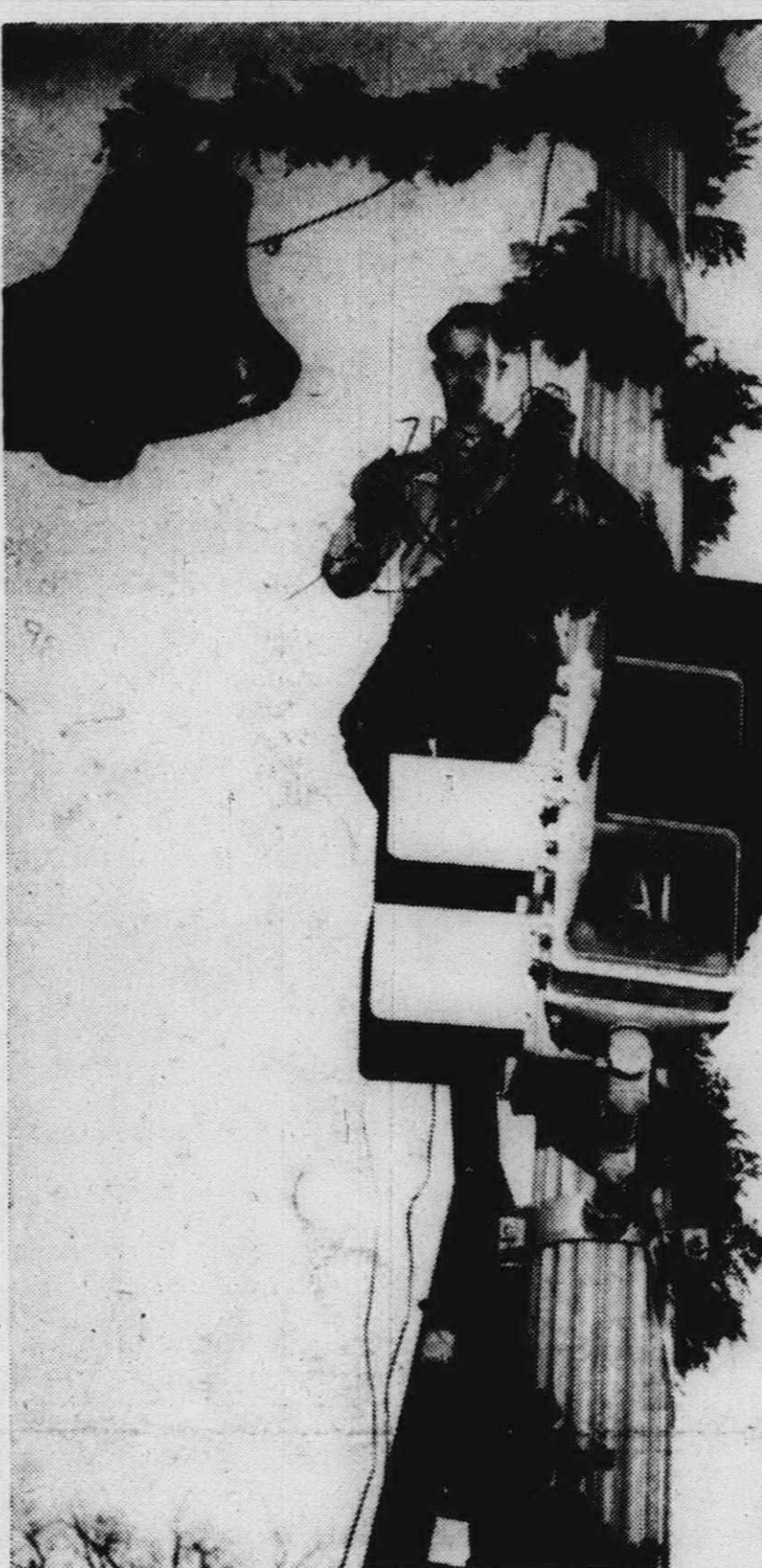
IT SEEMED MORE LIKE JUNE than December when City workmen put up Christmas decorations on lamp poles Monday. DPW worker Arlie Bagwell is shown working in the heat of the day (63 degrees!) at Main and Ann Arbor Trail. But by Tuesday it turned cold and snow covered the ground last night to finally make it look Christmas-like.
