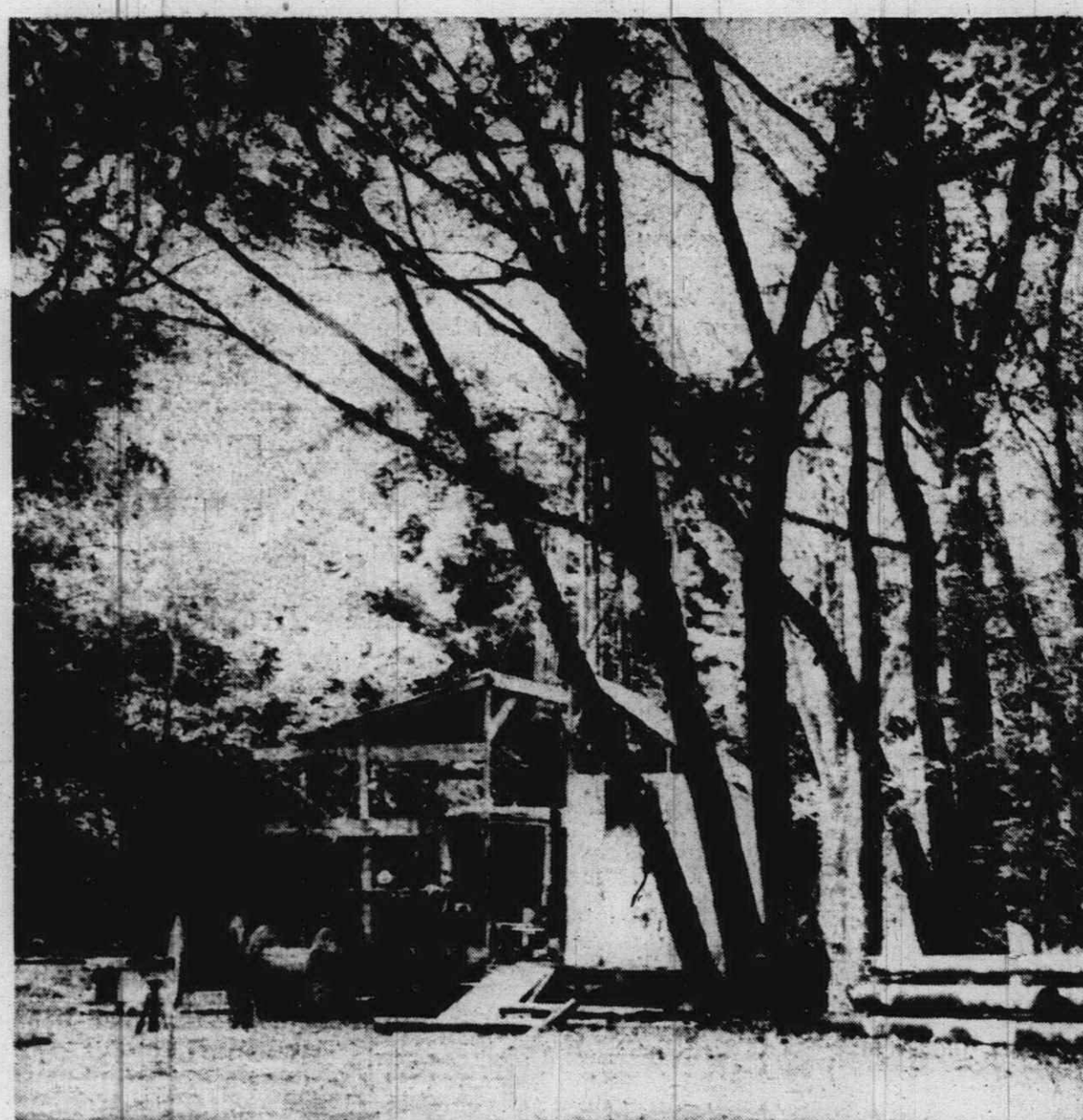
NESTLED IN a grove of trees overlooking Gunsolly Drive in Riverside Park is an oil rig that has been drilling for several months. Now down 3,653 feet, a trace of gas has been found. The objective should be reached in several days.
