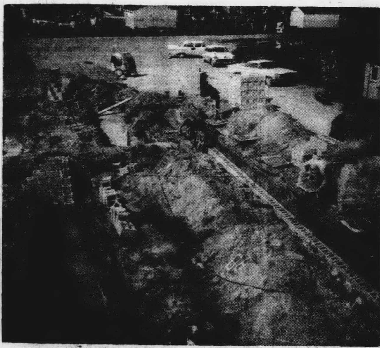
WORK HAS ALREADY started at Bird and Smith Elementary schools on additions that will provide more classrooms. Shown is Smith School where a new wing is being constructed on the north side of the building.
