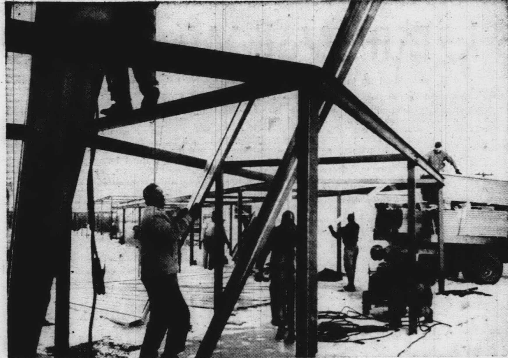
FIFTEEN MEN from the R.C. Mahon Co. of Detroit donated their time and the company the materials for covering a walk between buildings at Our Lady of Providence School on
