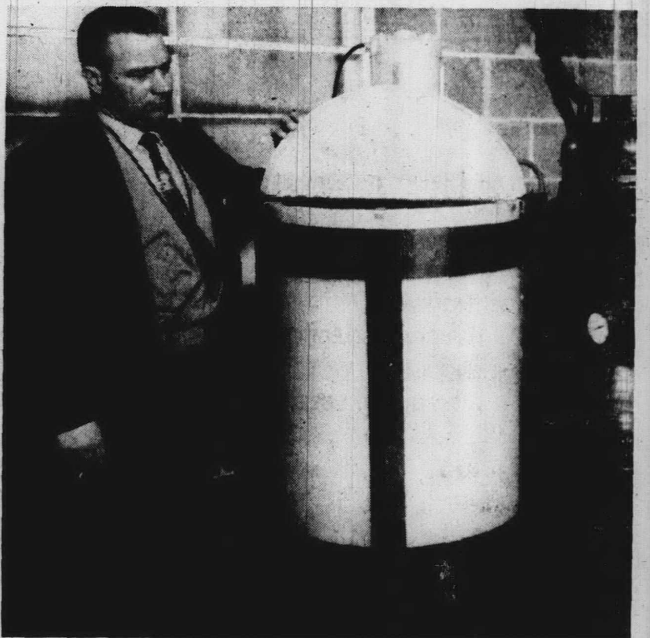
ONE OF FOUR dispensing units that will drop Calgon into the city's water supply is being examined by DPW Supt. Joseph Bida. The additive is tasteless and harmless to the body but is
