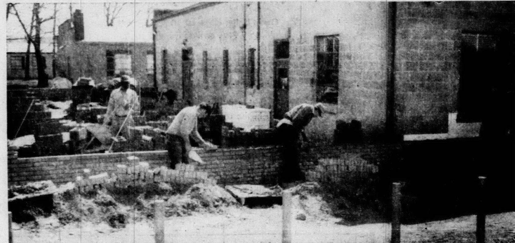
GROWING PLYMOUTH Township has affected Township Hall too where an addition is being built. Workmen are shown laying up the brick walls that will provide additional space for
