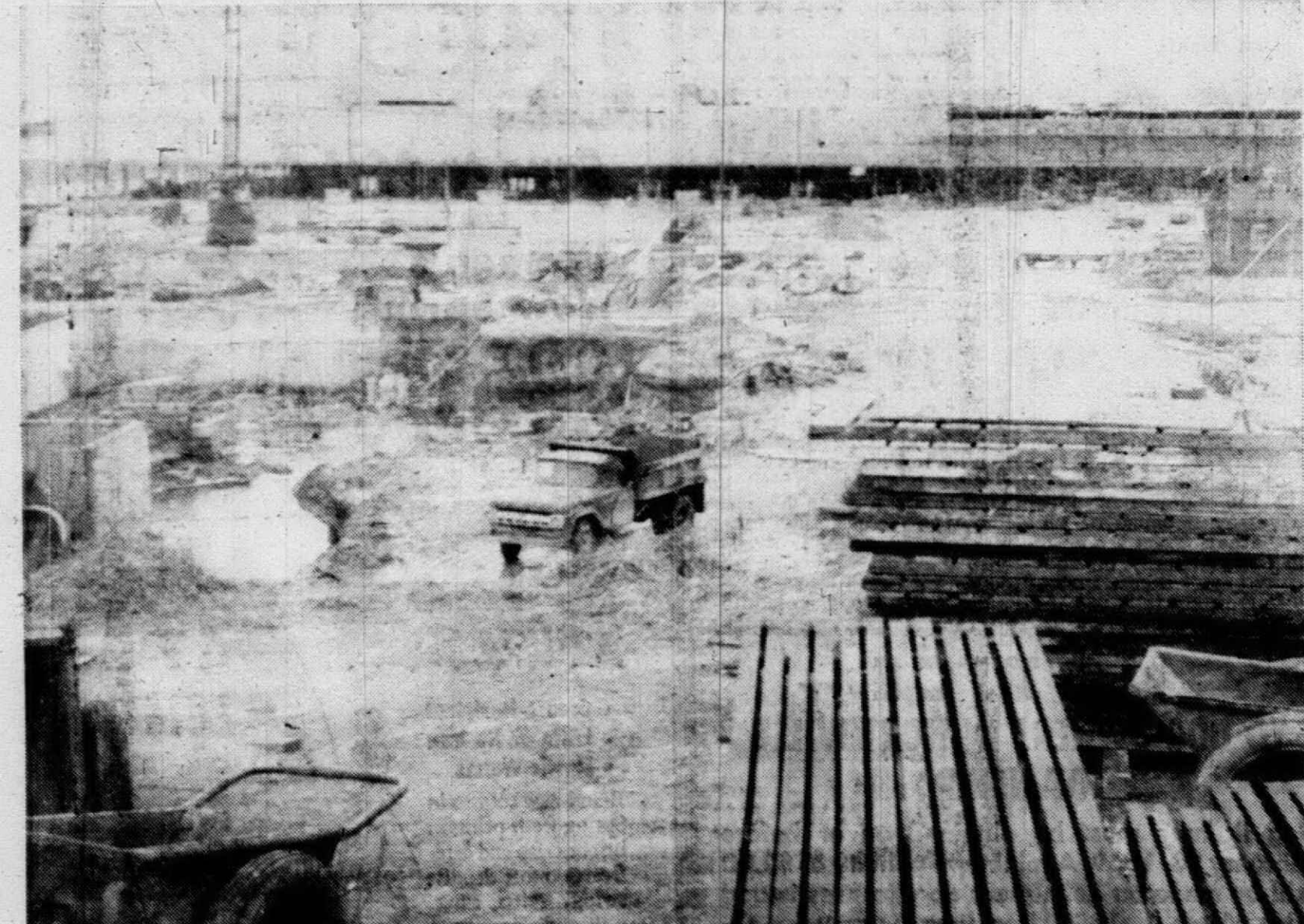
THIS VIEW LOOKING WEST from Montgomery Ward's shows basement excavations for two stores and the east wall of the big Federal Department store.
