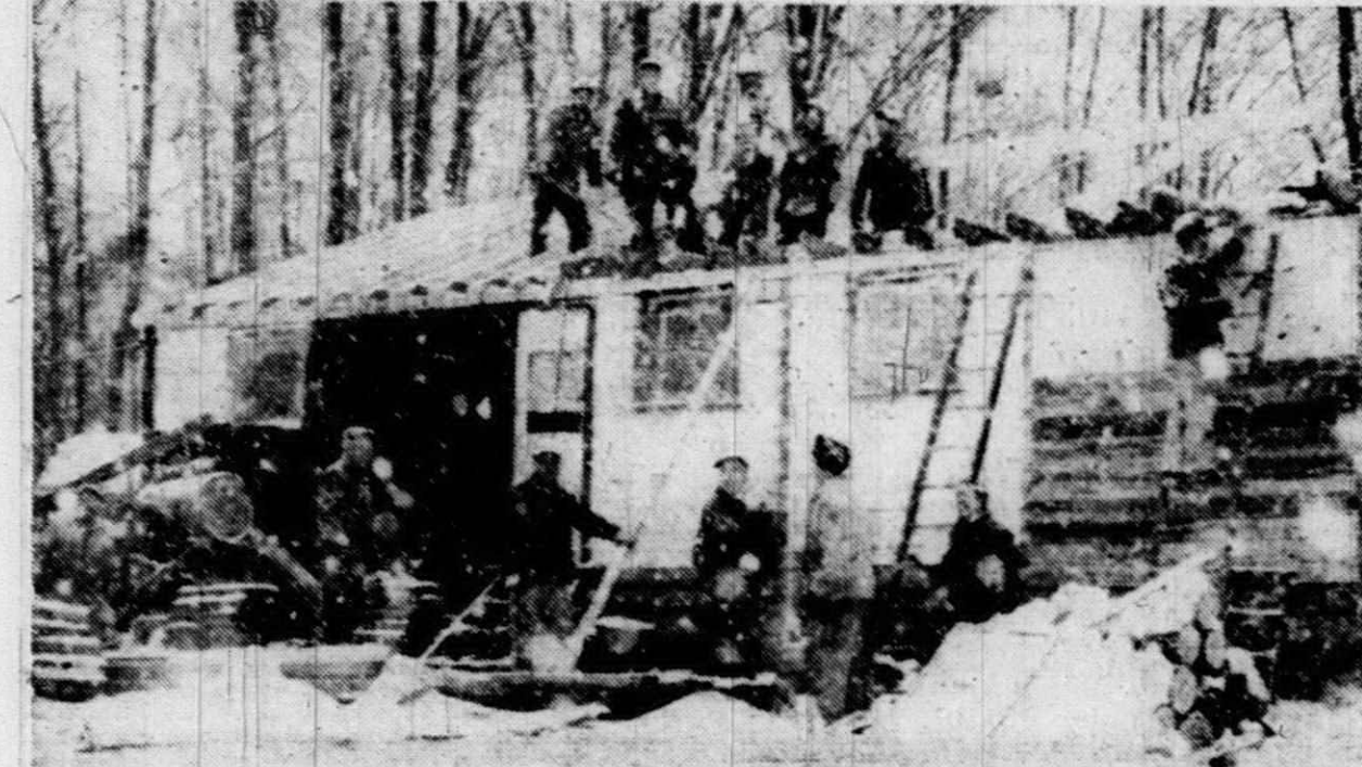
WEATHER WAS against the 18-20 men that struggled to put a roof on the William Tubert home at 1335 Lotz Road last Saturday
