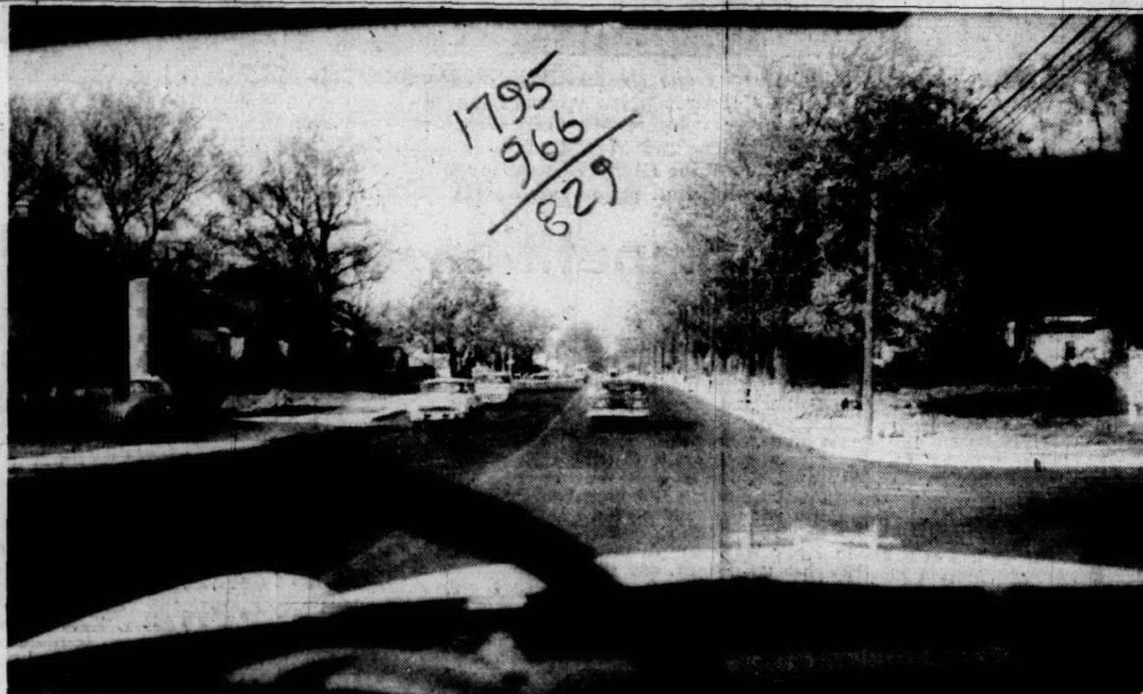
FINISHING TOUCHES are being given the South Main St. project which opened to traffic last Friday night. This picture is a driver's eye view of the four lane street. Some utility poles still need to be removed by Michigan Bell to finish the sidewalk. Ann Arbor Trail, from Main to Harvey, has been completed for a week. Sheldon Rd., from Ann Arbor Trail to the railroad, has one lane open most of the way and should be completely open sometime next week. Curb and gutter are being installed in Hough Park Subdivision but pavement will not be laid until next spring.
