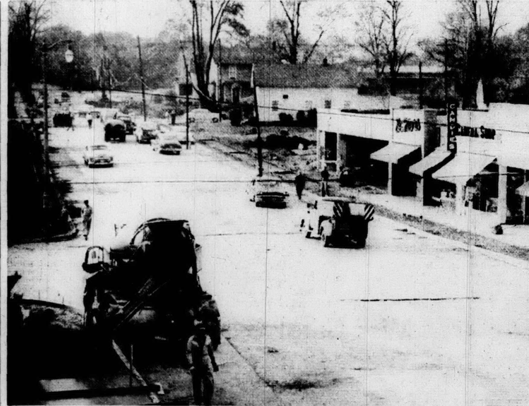
SIDEWALK SUPERINTENDENTS are having quite a season in Plymouth nowadays with three large projects going on at the same time. This is the widening and paving project of Ann Arbor Trail, from Main to Harvey. Other projects are South Main St. and Sheldon Rd. This shot, taken from the Mayflower Hotel, shows the pouring of sidewalks along the widened street. Concrete has been laid and asphalt is next.
