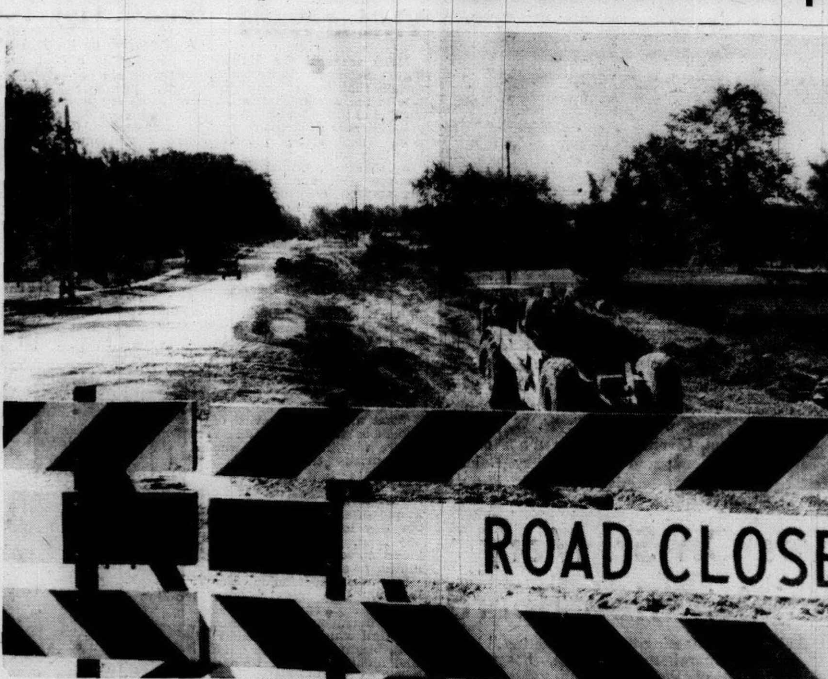
TWO MORE lanes are being added to Sheldon Rd. from the railroad to Ann Arbor Trail with work already well underway. The road is usually closed during the day and opened at night. City citizens along the route have protest-
