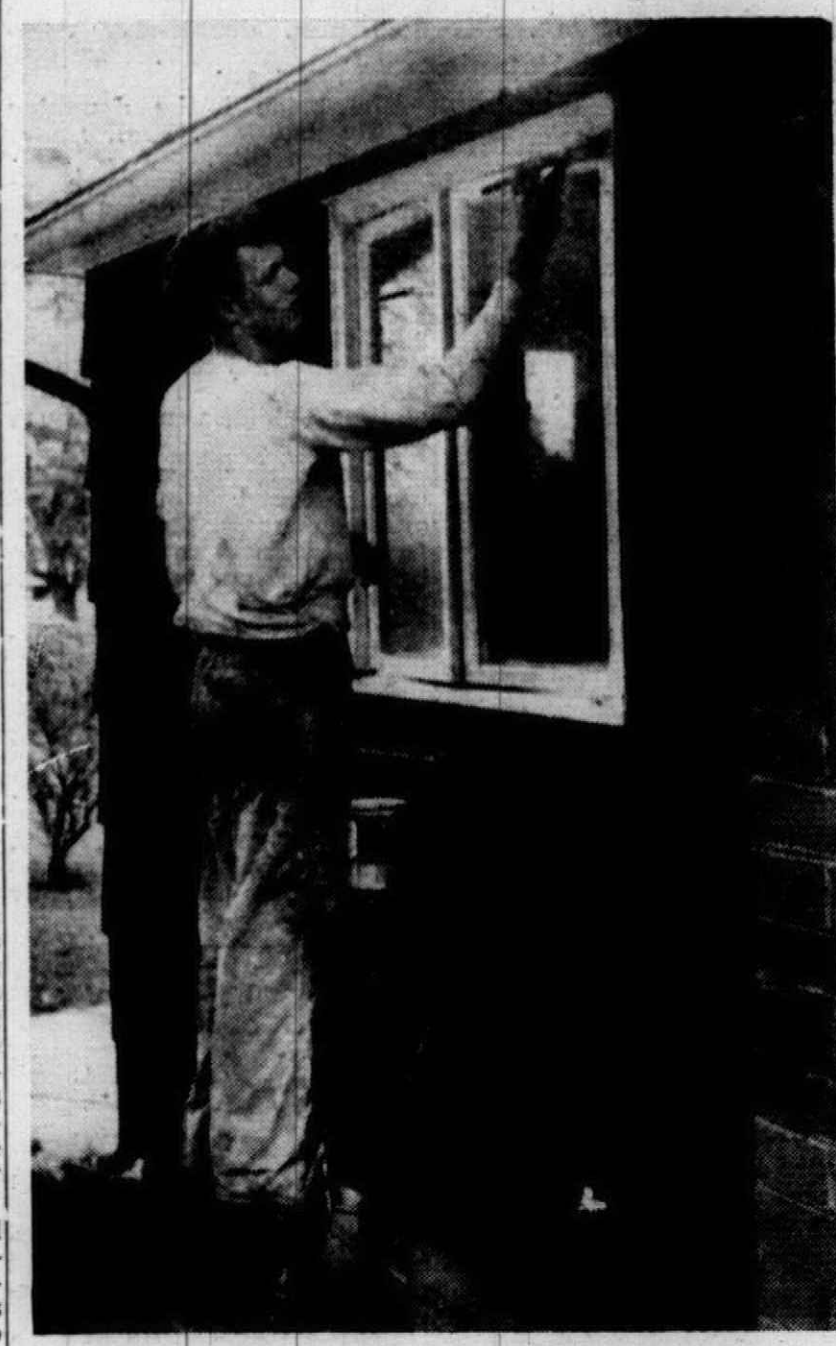
FALL PAINTING accomplishes more than a fresh exterior, if colors are chosen to accent a good feature of the house, minimize a poor one.
