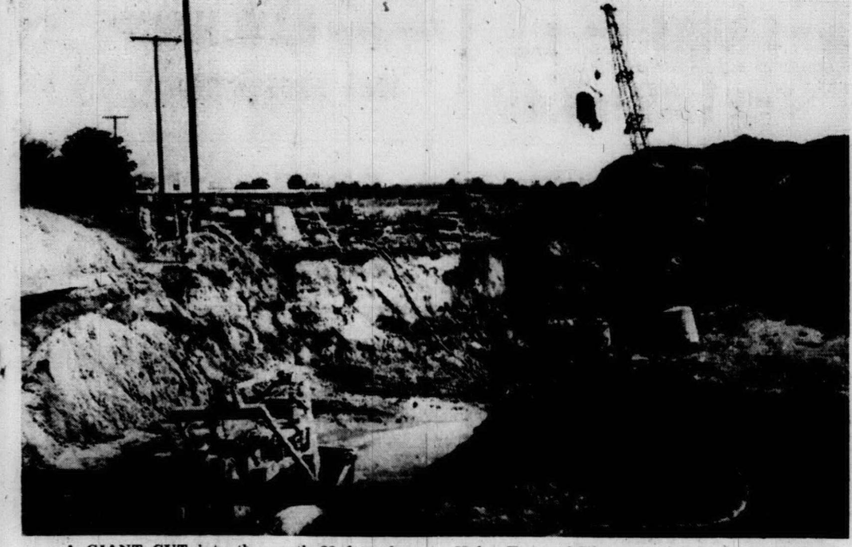
A GIANT CUT into the earth 28 feet deep has been made across Schoolcraft Rd. to accommodate a sanitary sewer that will service the new school opening next month.
