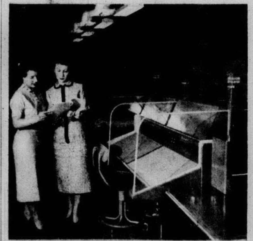
MARIAN SODITCH and Rosemary Comfort, Plymouth chief operator, stand near the latest type "information" switchboard in the new dial office.
