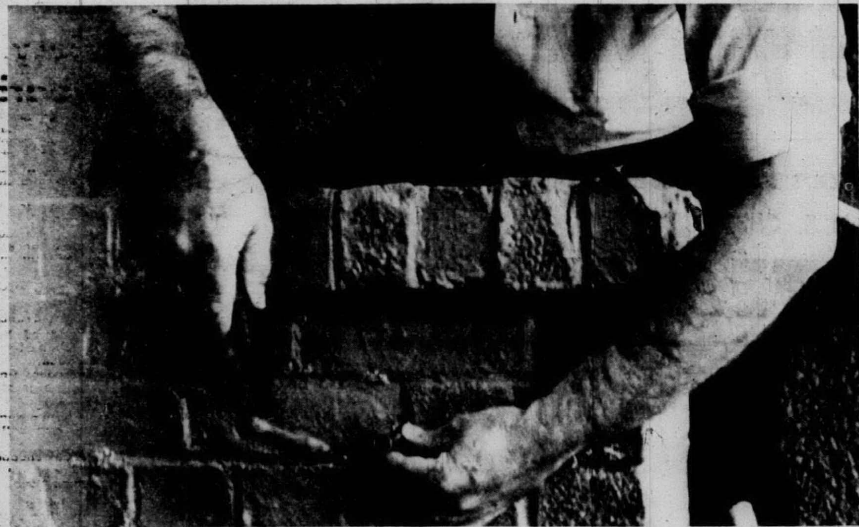
HALF-INCH copper or galvanized drain pipe is put in hole drilled previously with a star drill.
