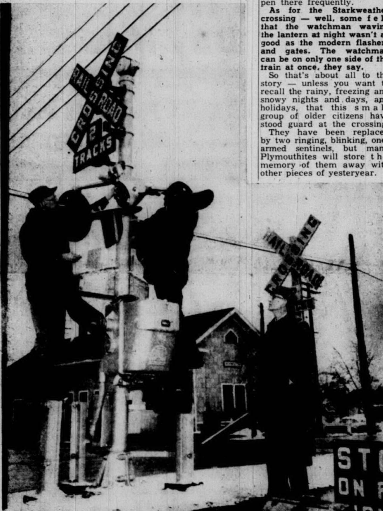
MODERN FLASHERS and gates took over the guard duties at Starkweather Ave. and Mill St. railroad crossings Tuesday afternoon. As workmen put up the flashers, Elza Baker, senior member of
