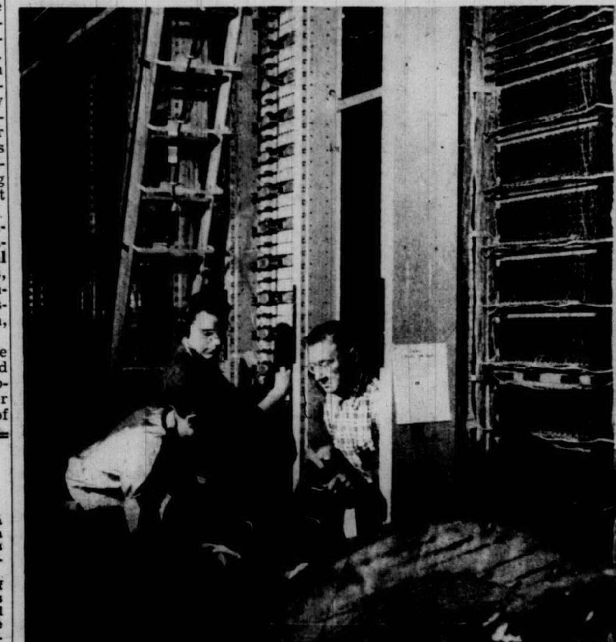
WESTERN ELECTRIC technicians are busy installing and testing the intricate telephone dial switching equipment scheduled for service
