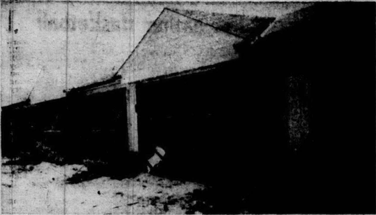
THIS IS a view of new apartments being built at the eastern end of Liberty St. A court is inside the
