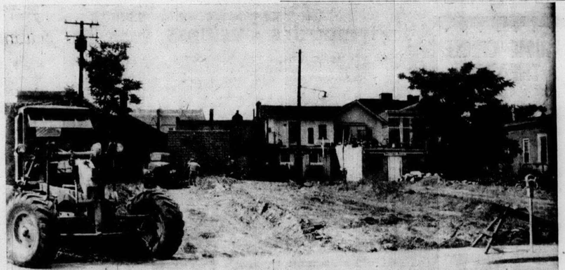
A NEW PARKING LOT for Plymouth was being readied for blacktopping this week. Located behind business establishments located on Penniman avenue and Main street, the paved lot will handle about 40
